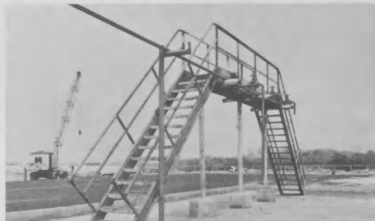
One of the new structures: a loading rack. Uno di e structuranan nobo: un loading rack.
